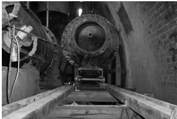
Fig 7: Valve on temporary rail system
